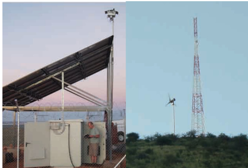
Figure 1: Wind/Solar Installation, Namibia Left: Solar Array, Battery, and Power Controller Right: Wind Turbine
