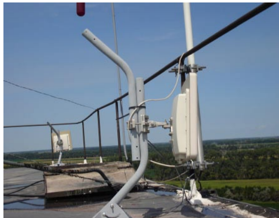
Located in Claremont, SD, this is one of five point-to-point links to the central server in Britton, carrying data and VoIP phone traffic for 4 Seasons Cooperative.
