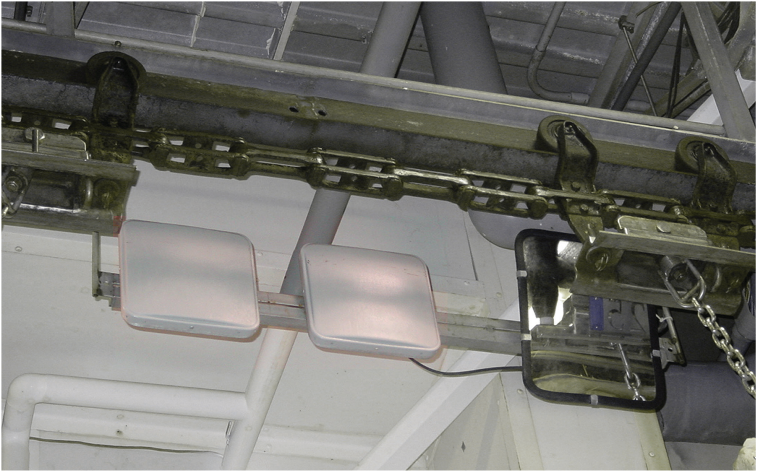
RFID antennas track and trace RFID-tagged food products as they move throughout the plant.
