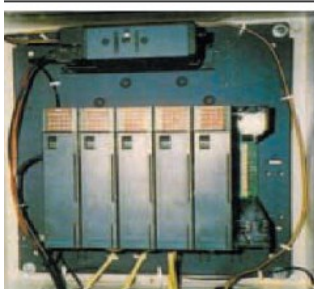
MOSCAD – Remote unit for Canal Gate & Rain Gauge Control.
