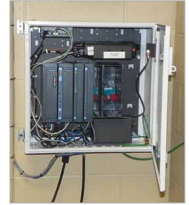
Remote Terminal Unit (RTU)
