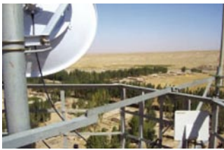
In Aqiang village, the PTP 400 Series bridge was installed with a dual-polarized antenna, 65 feet (20 meters) high.
